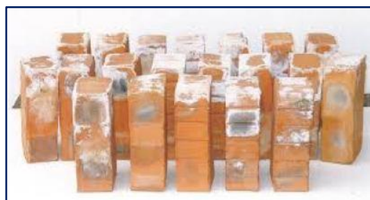
Figure 6: Efflorescence on Bricks
